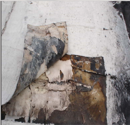
Roof damage requiring immediate repair
